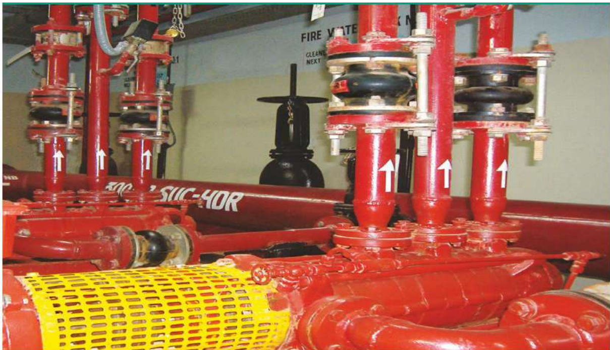
Fig: - Typical Pic of Multi Stage Multi Outlet Fire Pump
